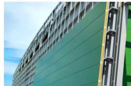
Application in Buildings
